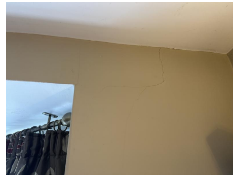
Photo 10 - Cracking above bay window.
