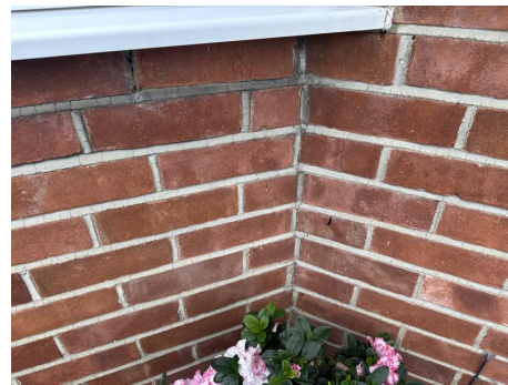
Photo 4 - Cracking to front bay.
