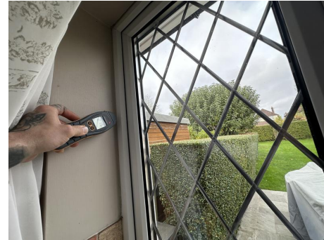
Photo 8 - Damp to side of kitchen window.
