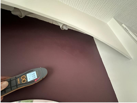
Photo 11 - Damp to bedroom one chimney breast.
