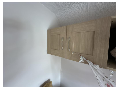
Photo 6 - Cracking to corner, bedroom two.
