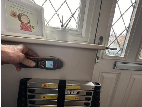
Photo 7 - Damp below front door window sill.
