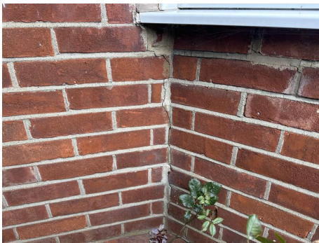
Photo 3 - Cracking to front bay.
