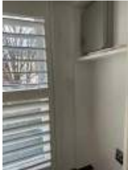
Photo 106 - Damaged finishes in utility room
