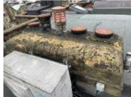
Photo 20 - Cracked render and no ventilation to the covered chimney flues
