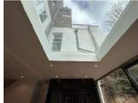
Photo 103 - dampness around rooflight
