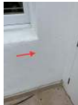
Photo 52 - Minor cracking to render
