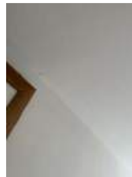
Photo 99 - Damp staining to the top floor landing
