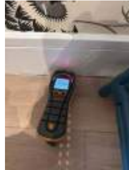
Photo 136 - Dampness found- lower ground
