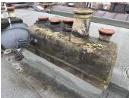
Photo 21 - Cracked render and no ventilation to the covered chimney flues
