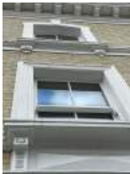
Photo 61 - Cracking to rendered window reveals and sills
