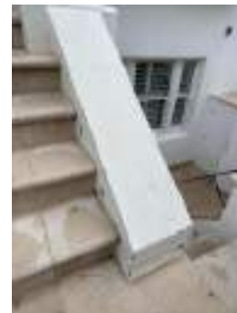
Photo 82 - Weathered and slightly cracked
