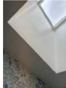
Photo 95 - Staining around skylight
