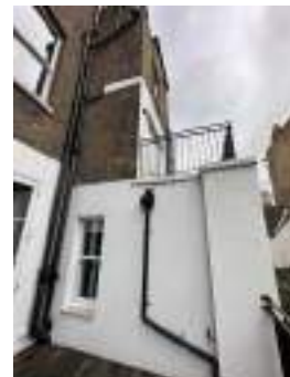
Photo 34 - Copings do not project sufficiently
