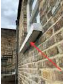
Photo 47 - Lack of drip grooves below windowsill
