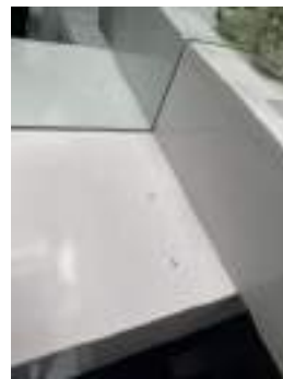
Photo 130 - Staining around worktop, wash-basin
