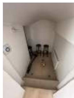
Photo 142 - Dampness to vault
