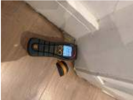
Photo 135 - Dampness found- lower ground
