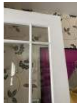
Photo 122 - Cracked pane and no safety glass
