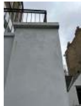
Photo 60 - Cracking and blistering to render
