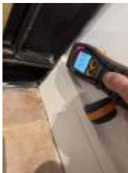
Photo 137 - Dampness found- lower ground
