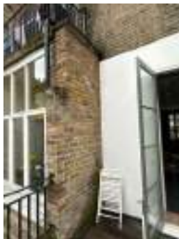
Photo 59 - Staining to wall caused by neighbours
