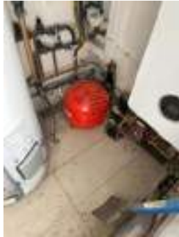
Photo 89 - Dampness and water
