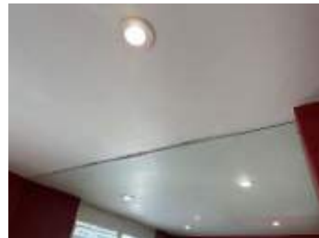
Photo 101 - Dampness to ceiling
