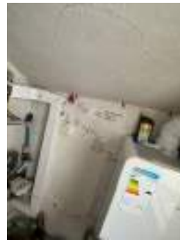
Photo 92 - Cracking to render
