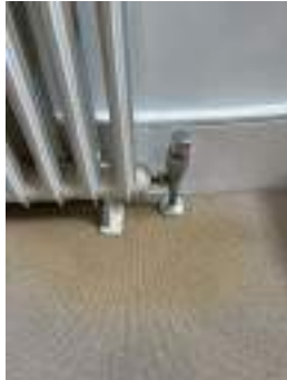
Photo 151 - Staining around radiator
