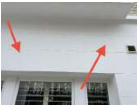
Photo 51 - Minor cracking to render
