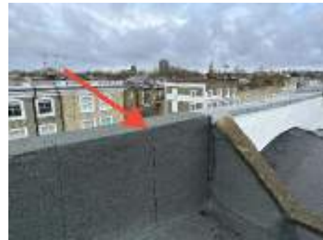
Photo 30 - No lead capping
