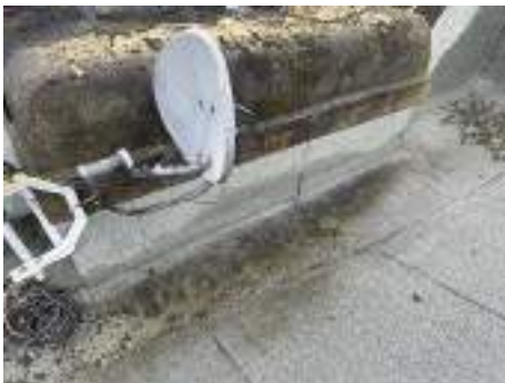
Photo 24 - Felt flashings, not as good as lead flashings
