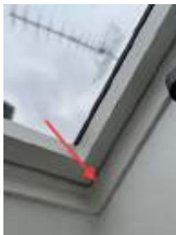
Photo 6 - Skylight has been sealed internally with silicon
