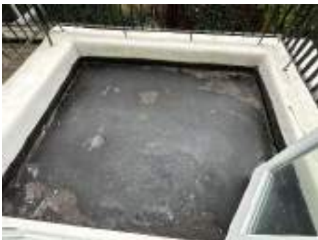
Photo 14 - Cracking to asphalt roof
