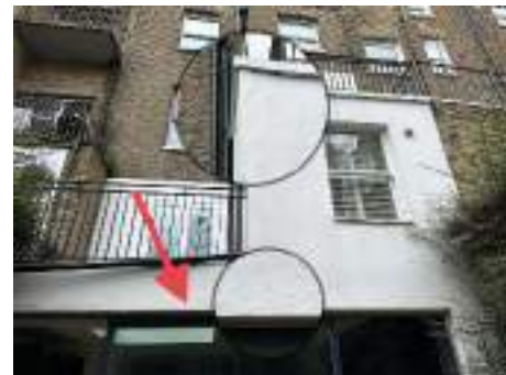
Photo 54 - Areas of cracking and blistering to the rear render
