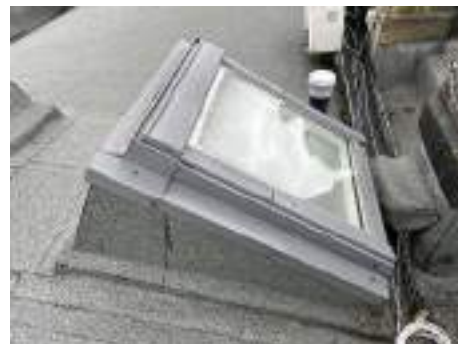
Photo 7 - Skylight potentially leaking requiring repair/ replacement
