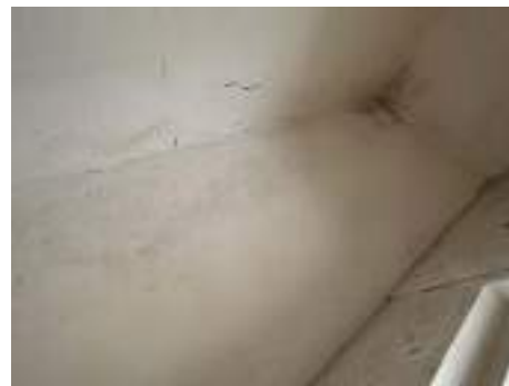
Photo 140 - Dampness to utility room ceiling void
