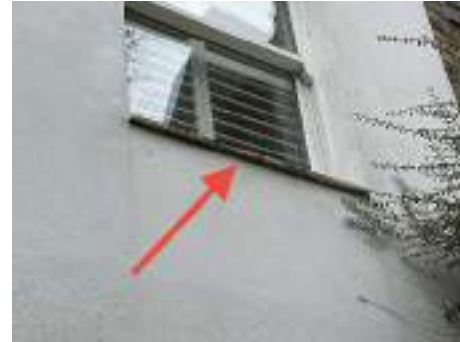
Photo 56 - Windowsill does not project sufficiently
