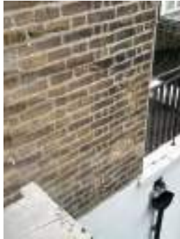
Photo 63 - Minor cracking to walls
