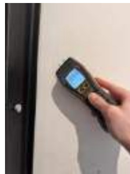
Photo 138 - Dampness found- lower ground
