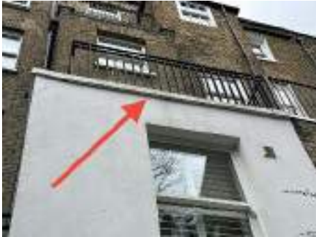
Photo 55 - Copings do not project sufficiently
