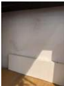
Photo 139 - Dampness found- lower ground
