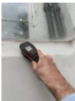
Photo 141 - Dampness due to rooflight leak
