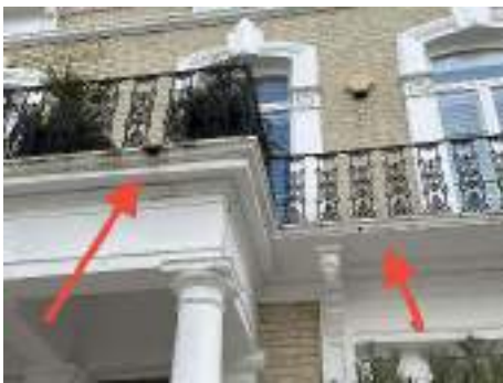
Photo 49 - Water staining as no drip grooves or cappings
