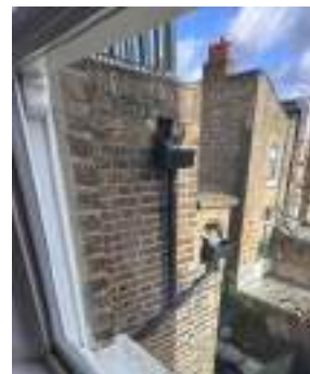
Photo 32 - No coping stones
