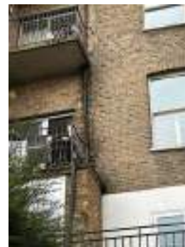
Photo 58 - Water staining to walls caused by neighbours downpipe
