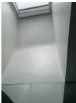
Photo 98 - Past staining from skylight
