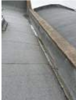
Photo 4 - Moss buildup and standing water
