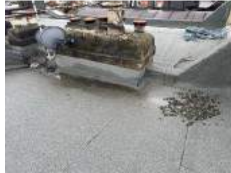
Photo 5 - Moss buildup and standing water
