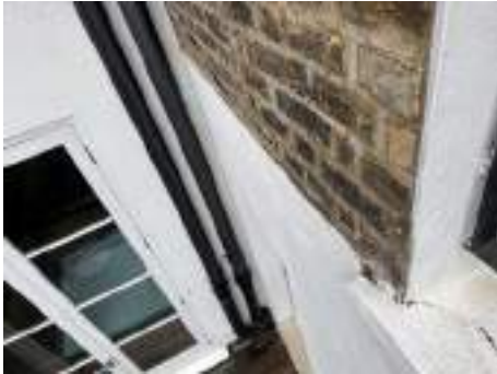
Photo 143 - Dampness possibly entering via ledge of render
