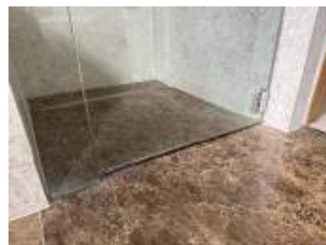
Photo 134 - Defective shower door seal
