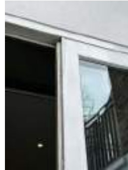
Photo 75 - Weathering and cracking to joinery
