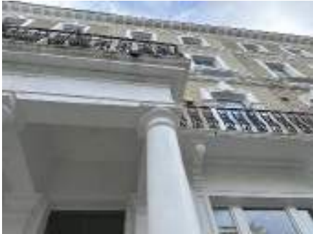
Photo 11 - Water staining and blistering beneath the balcony and portico
