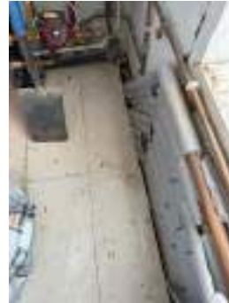
Photo 90 - Loose and cracked flooring
