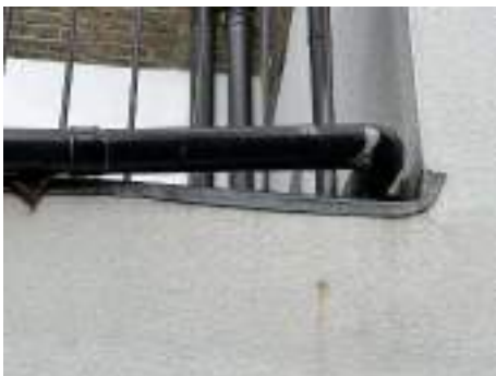
Photo 41 - Stained joints, repaired
