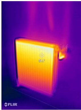
Figure 5- Thermal imaging shows radiators heat up
